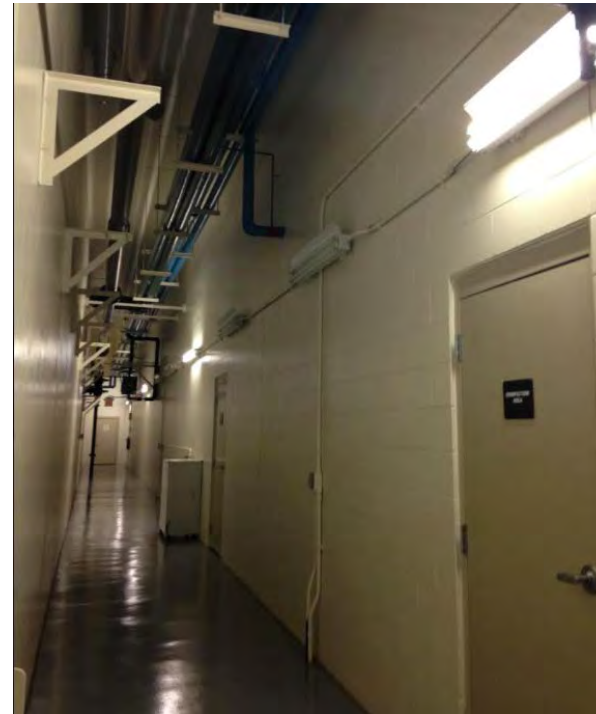
Main hall lighting
